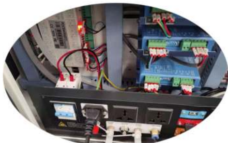
Control cabinet with RD laserword
